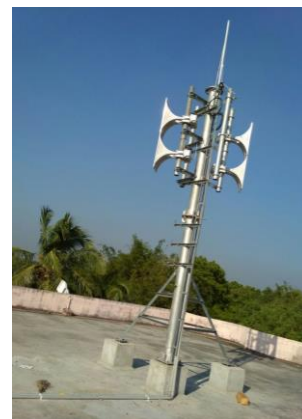
Roof Top Pole 5 Mtrs – 57 Nos.
