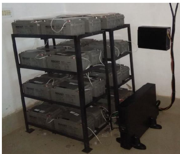
UPS with Battery Bank
