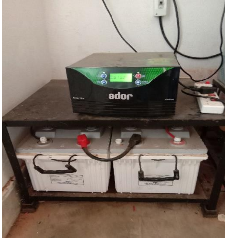
Solar Inverter & Batteries
