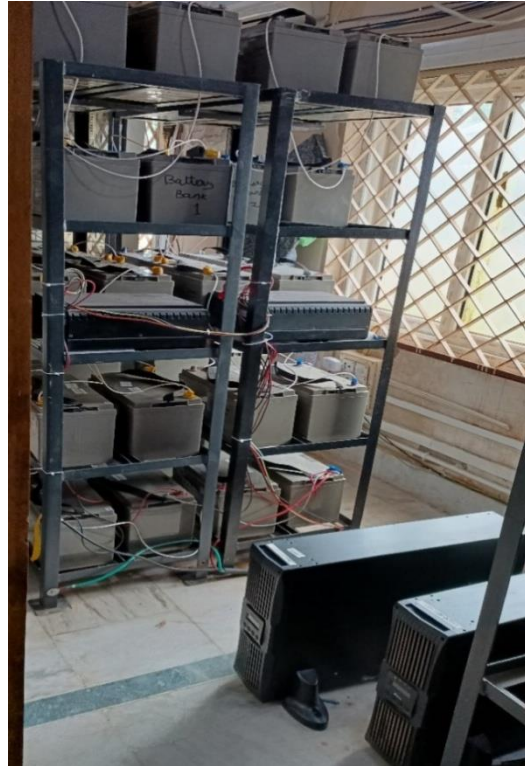
UPS & Battery Bank
