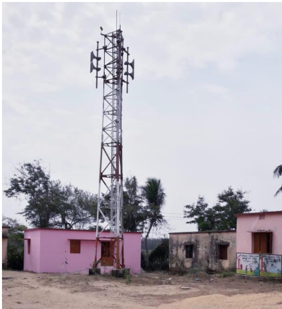
Metal Angular Tower
