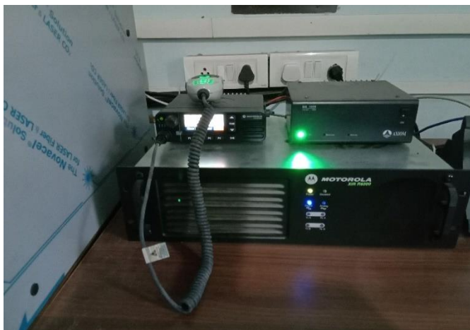
DMR Repeater and Fixed Station
